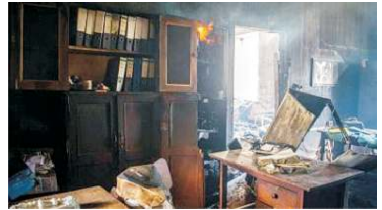
A fire remains inside the burnt building at the Ivory Tower of Makerere University in Kampala on September 20, 2020. - Copyright © africanews BADRU KATUMBA/AFP or licensors
